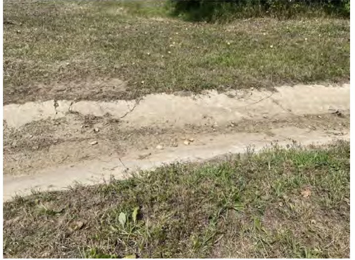
Outfall drainage trench – Minor damage from mower
