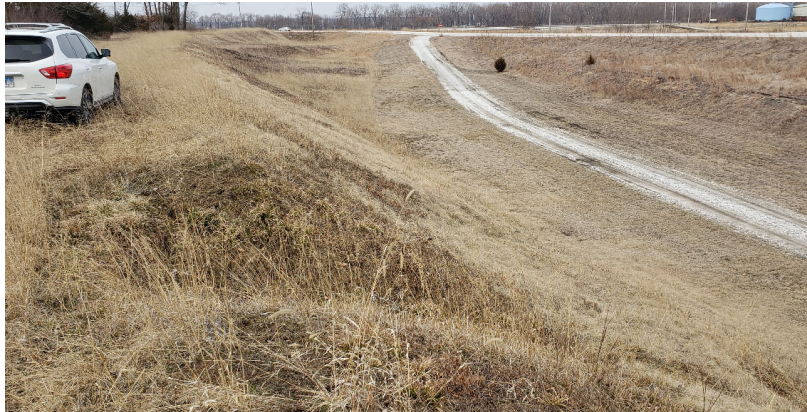
Old East Pond Berm washout
