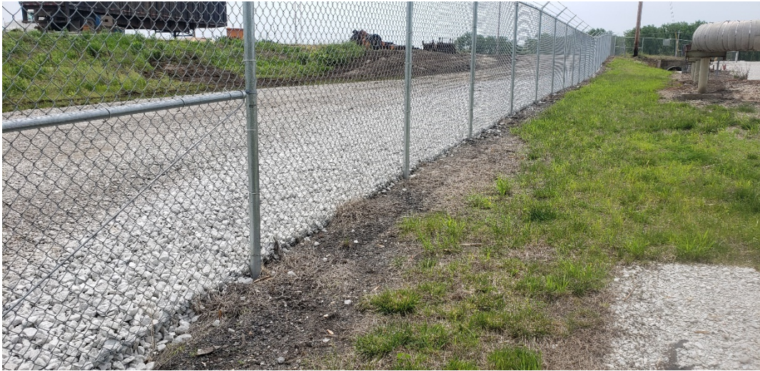
REPAIRED MAY 2022 - Minor soil washout under the fence by well 9
