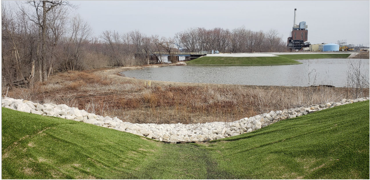
Fly Ash Pond Cap – outlet 5; Bottom Ash Cap - west side berm view
