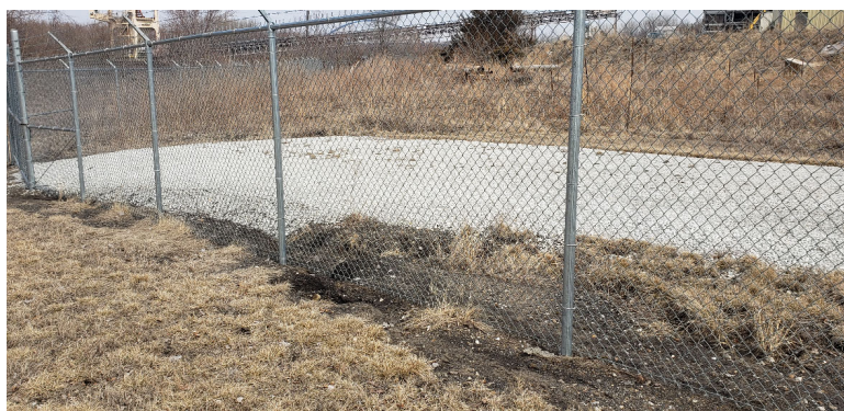
Minor soil washout under the fence by well 9
