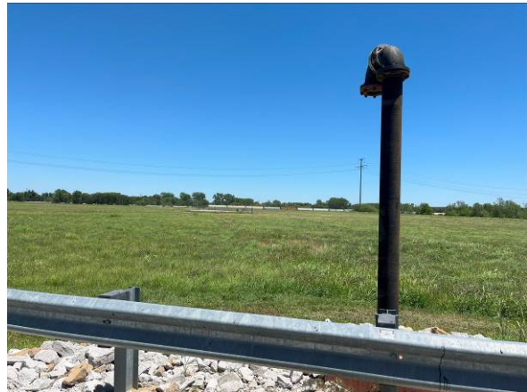
South Pump station, facing east
