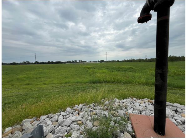
South Pump station, facing east
