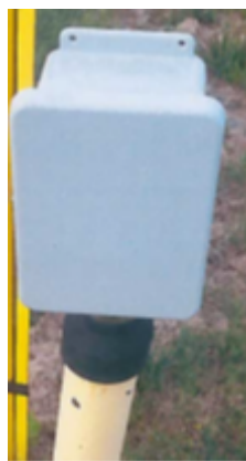
Enclosure for Probe, Cable, and Connector
