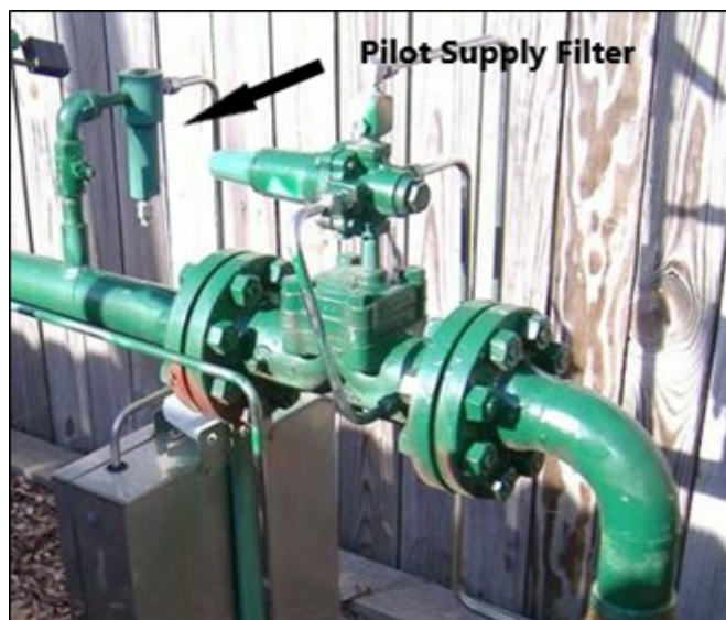
Figure 2: Pilot Supply Filter
