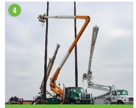
4 Aerial H-frame assembly. Ground framing may also be utilized prior to drilling and setting poles.
