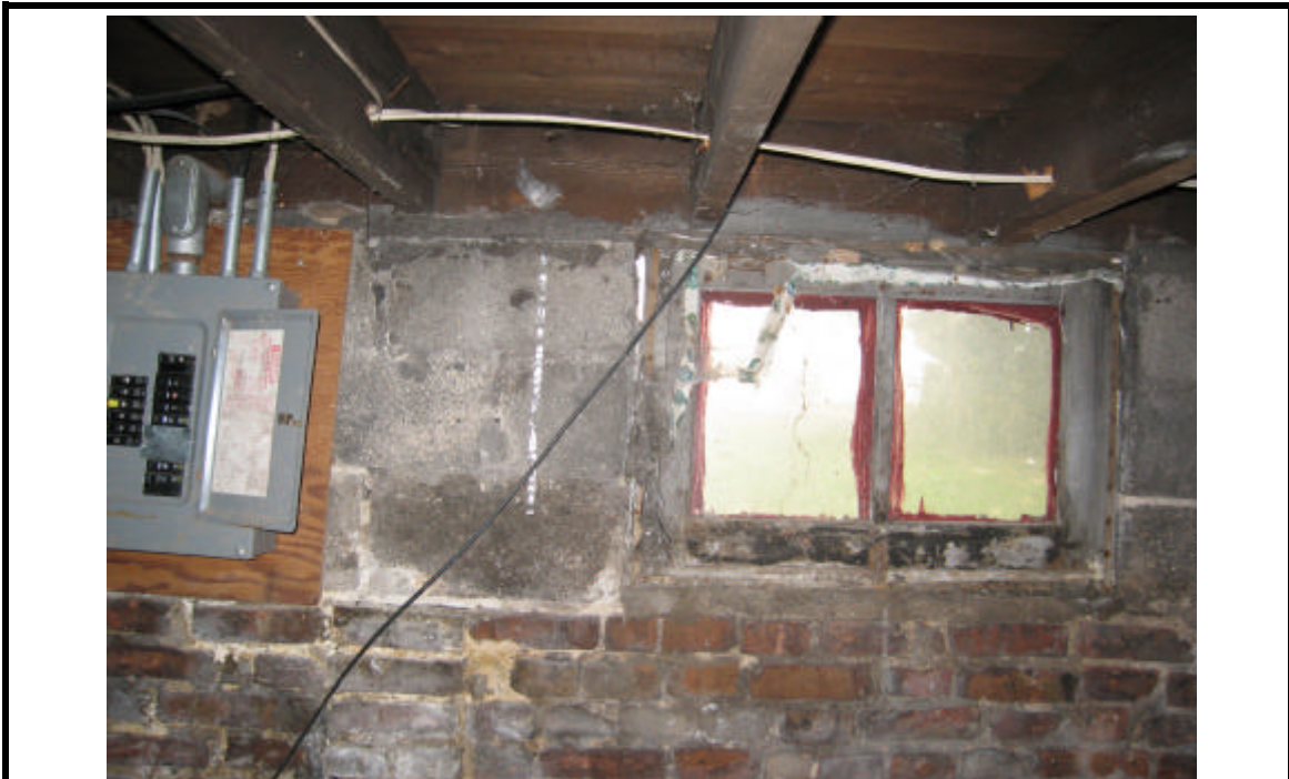
PHOTO 15: View of window along south wall of basement. There are several gaps between window frame and bricks & cinder blocks in this area and throughout basement.
