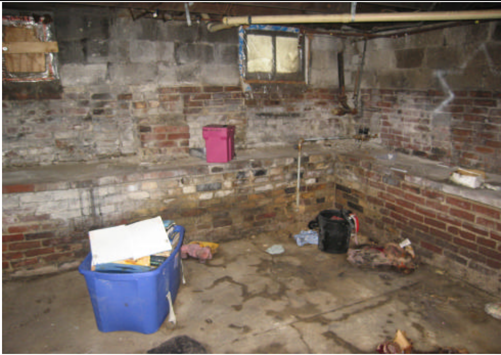
PHOTO 13: View of small basement room looking SE at corner of room. Left wall is outside east wall and right wall is interior wall with crawl space beyond.
