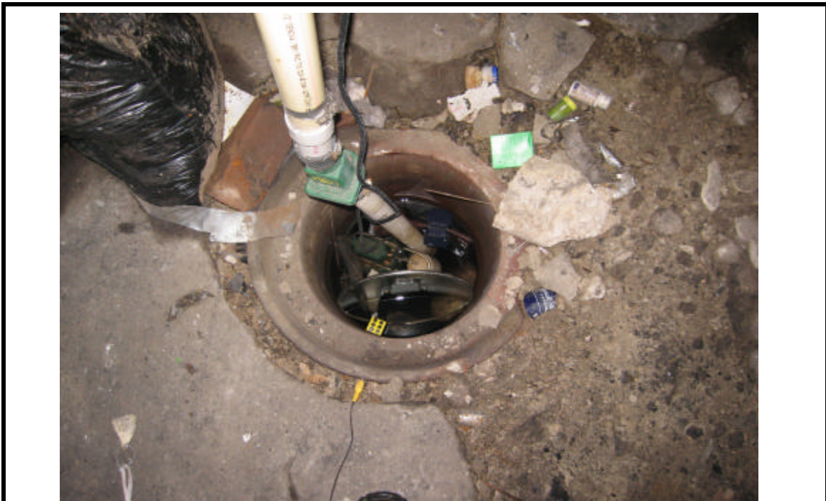
PHOTO 12: Inside basement of 507 E. Washington looking at water in swamp. Note broken concrete floor slab and exposed soil.
