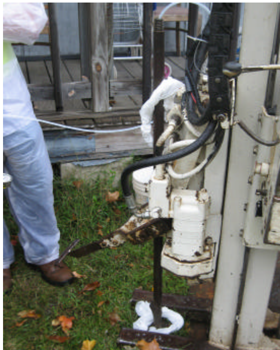
PHOTO 8: Another view of leak detector paper towels around rod on top of bentonite putty seal at VP412EHill-3 location.
