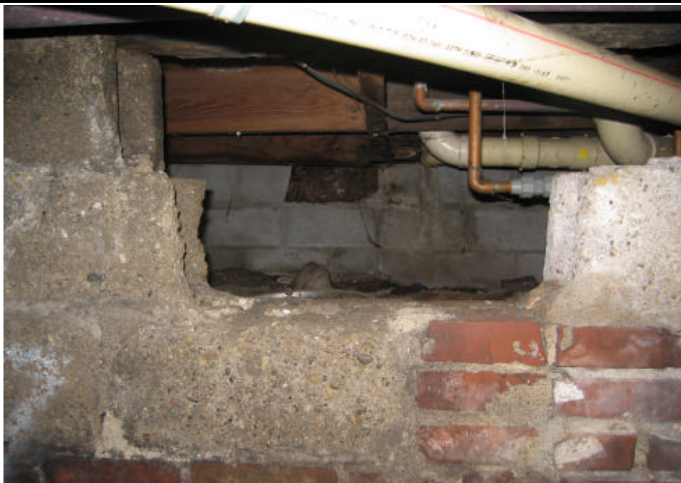
PHOTO 14: View from small basement room into crawl space below northeast corner of house.
