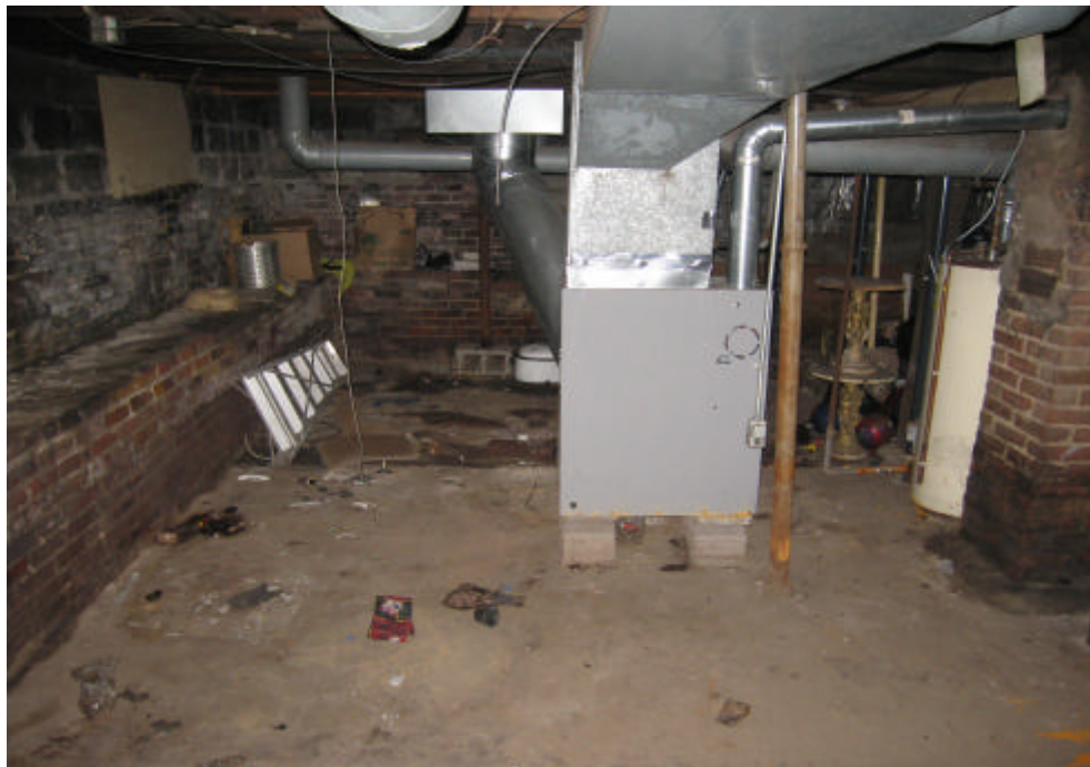
PHOTO 10: Inside basement of 507 E. Washington looking east along north wall. Note new central heating unit and water heater, both fueled by natural gas.
