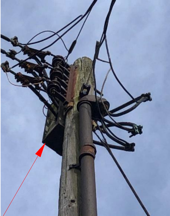
Elevated (bird cage) CT Metering On a Meter Pole
