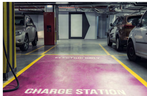
Multi-Family Dwelling Charging
