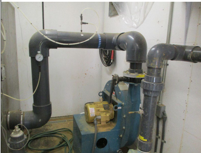
Photo #: 3 Taken by: Maher, Christopher Entity: Huster Substation Permit: MO0137642 Location: Treatment Building Description: Air blower motor for air stripper system. Date Taken: 11/3/2023 Media: WPC
