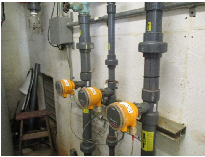
Photo #: 1 Taken by: Maher, Christopher Entity: Huster Substation Permit: MO0137642 Location: Treatment Building Description: Meters for flow from three extraction wells. Date Taken: 11/3/2023 Media: WPC
