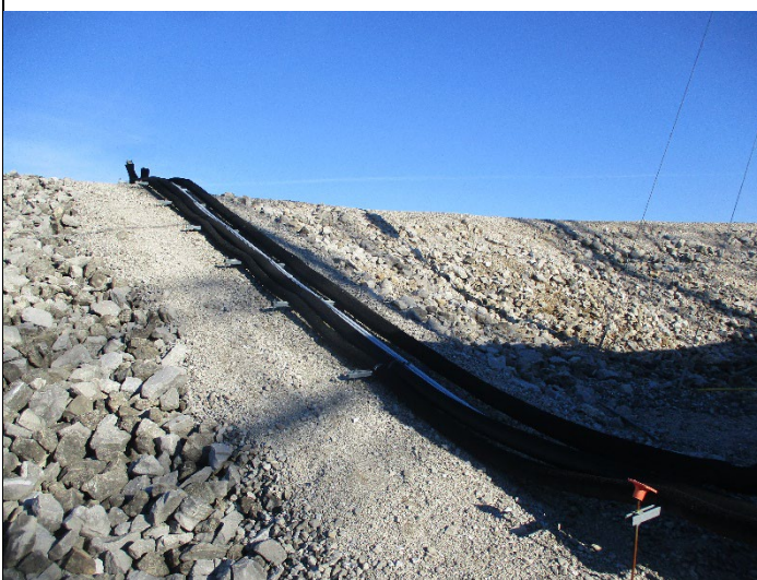
Photo #: 5 Taken by: Maher, Christopher Entity: Huster Substation Permit: MO0137642 Location: Near Treatment Building at Levee Description: Effluent line on right side and influent line over levee berm; facing north. Date Taken: 11/3/2023 Media: WPC
